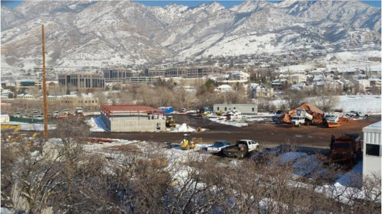
Figure 2- The yard is busy as crews move in and out during work throughout the day.
