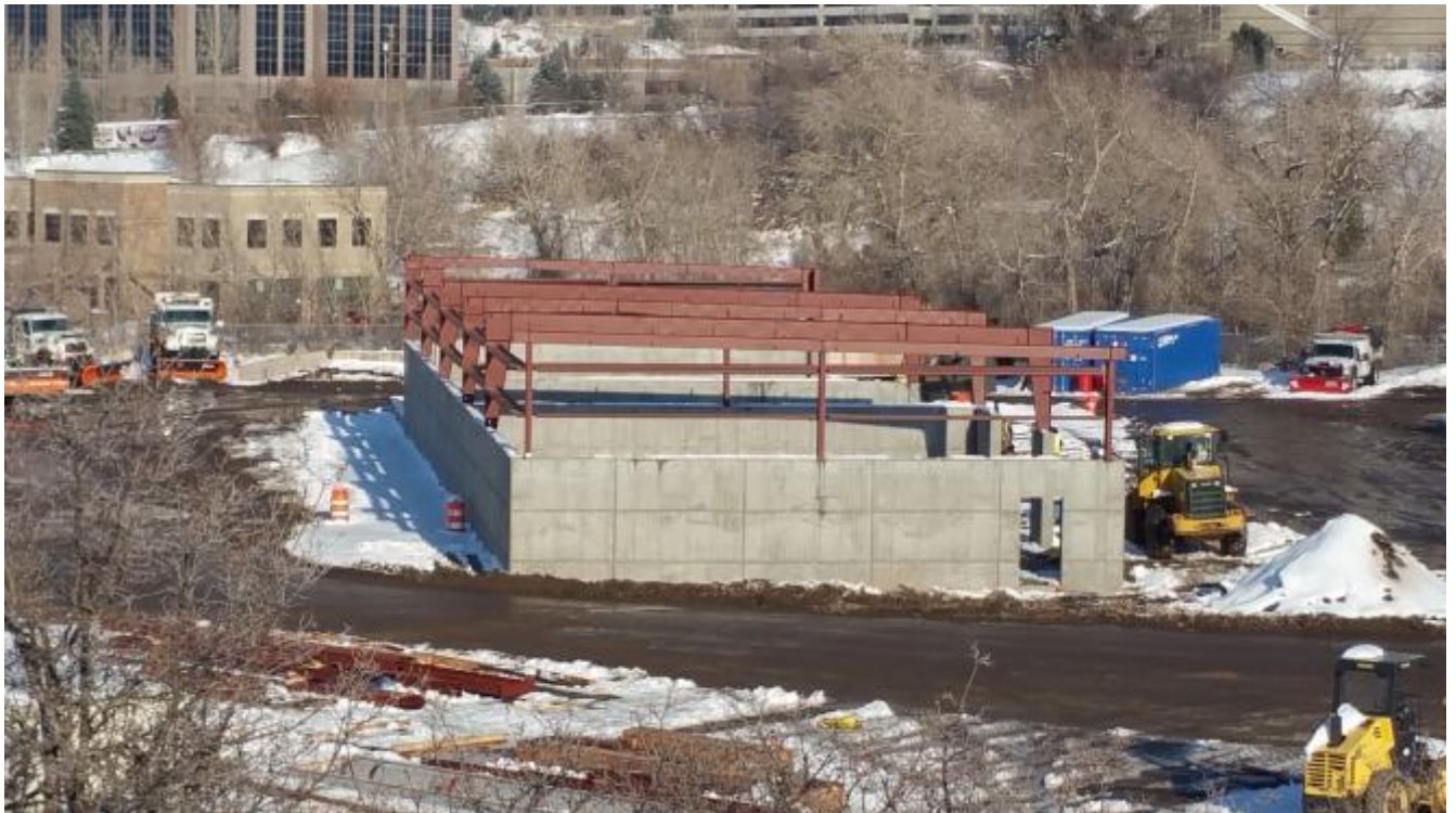
Figure 1- The steel structure is going up on the public works salt shed.
