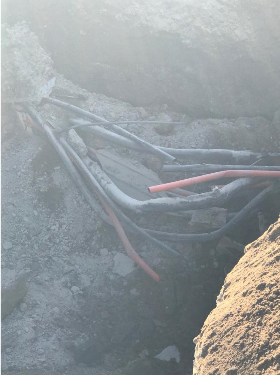
Figure 1- Due to an error in marking the communications utility conduits by Blue Stakes (not marking), the contractor installing the storm drain line broke the conduit banks and the cables (1800 pair, 1600 pair, 800 pair, fiber optic, etc....). 2300 East will be closed during the repairs for safety reasons.
